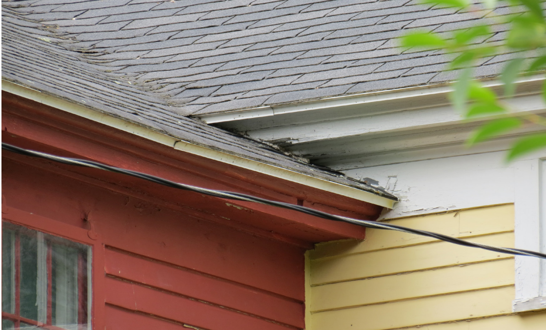
Detail view of the valley where the roofs of the two sections of the house meet. Water flowing down this valley and from the ell roof contribute significantly to the water issues on the rear wall of the 1814 house (yellow wall). A gutter previously installed here to mitigate the issue has fallen to the ground. SCC, July 2019.
