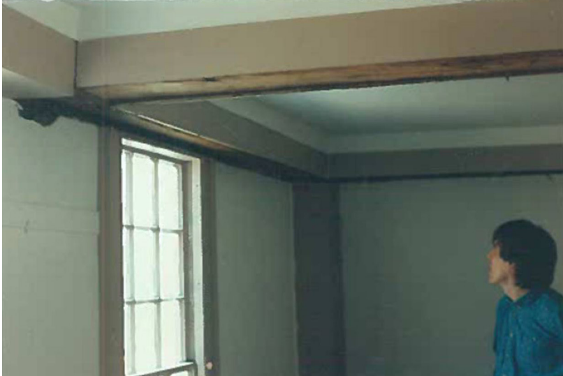
This 1990's view shows that only the bottoms of most of the beams were exposed, making it impossible to detect deterioration in the tops of the beams unless it extended all the way to the bottom.
