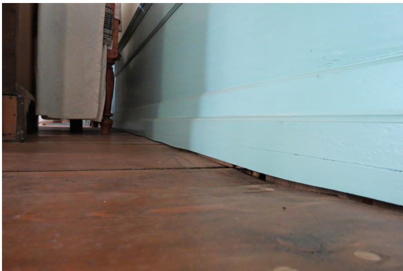
Another view of the sagging floor and previously altered baseboard. Note wood plugs in floorboard in foreground, which cover screws installed after the 1993 repairs. SCC, July 2019.
