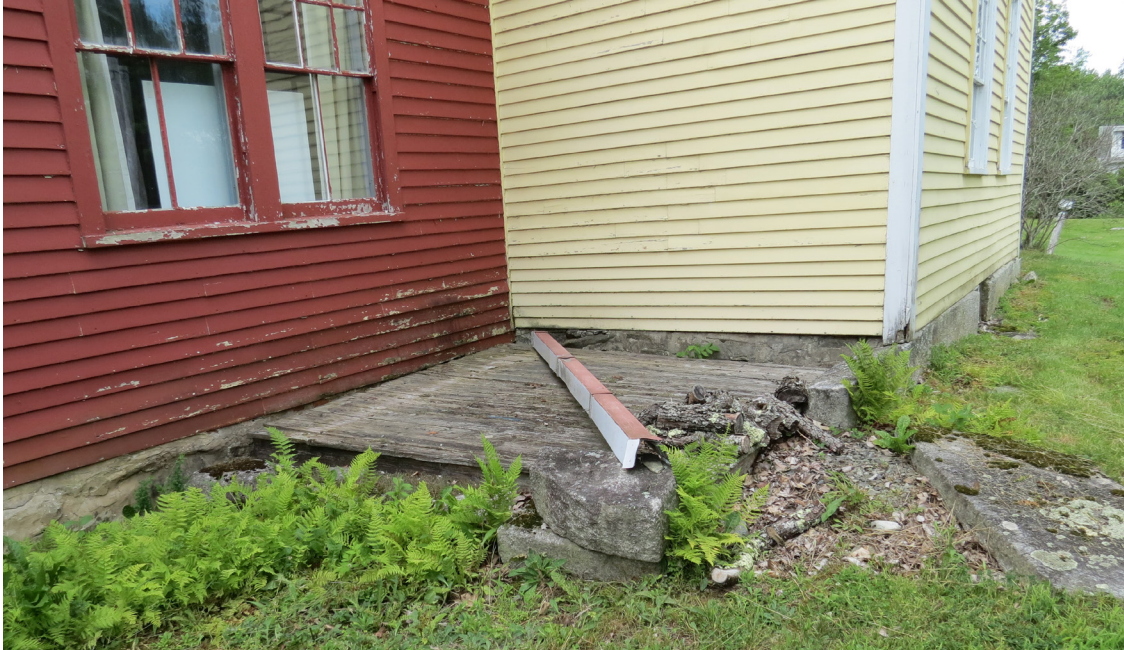
Current conditions in the northeast corner where the 1814 house (yellow) is joined by the 1896 ell (red). The buttery/cheese room built in 1814 stood where the wood platform is located. Note the fallen gutter, which was installed on the roof of the ell at some point after 1993. SCC, July 2019.
