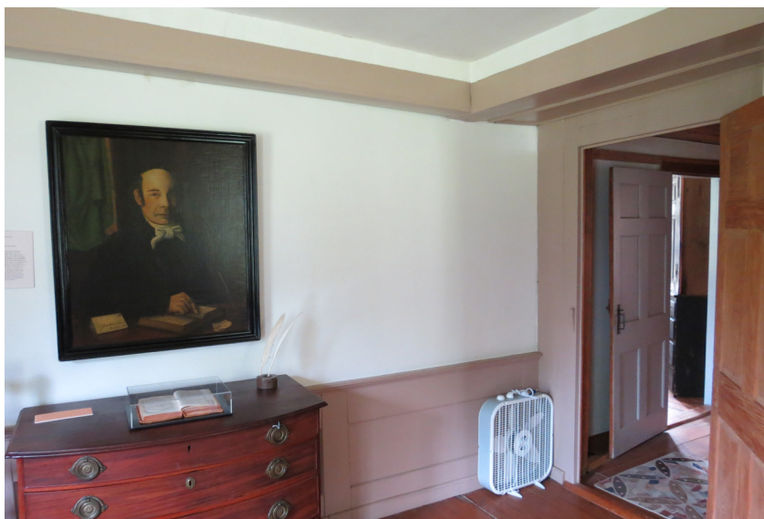
Current view in parlor of the area below the sagging floor. Wainscot and plaster adjacent to the door at right was installed to cover original door opening, apparently during 1950's restoration. SCC, July 2019.
